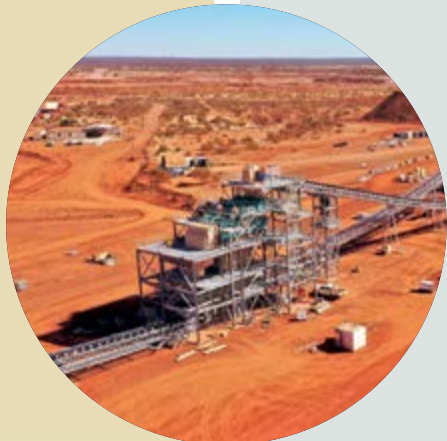
MACA Interquip awarded engineering, procurement and construction management contract for Tomingley Gold Operation
